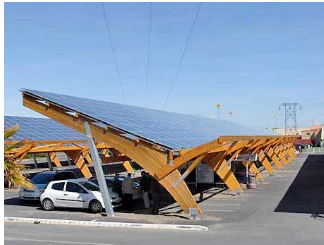
Figure 14 : Ombrières de parking photovoltaïques (Montpellier)
